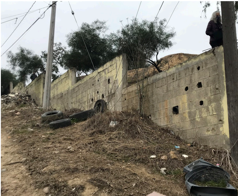
Collapsing perimeter wall Portions of the perimeter wall are redesigned in the proposed plan.
