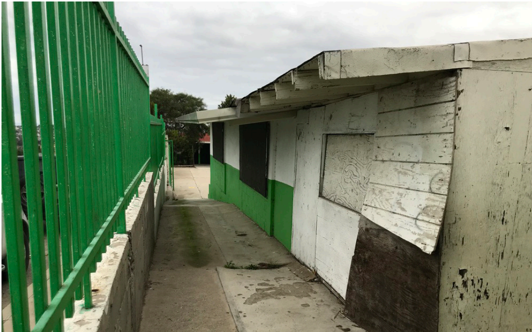
Boarded-up structures on the campus These delapidated structures need to be rebuilt
