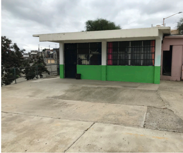
Unusable structures at the edge of the main space Several structures are beyond repair. Some materials may be reusable.
